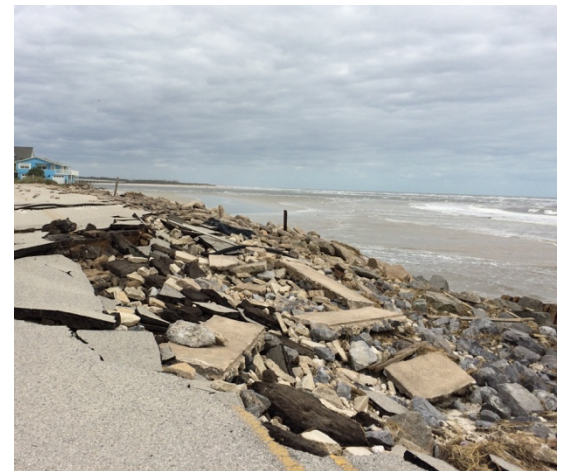
Photo (above): Damage on Highway A1A near St. Johns County, Florida after Hurricane Matthew. Photo by Eileen Lainez (October 2016).
