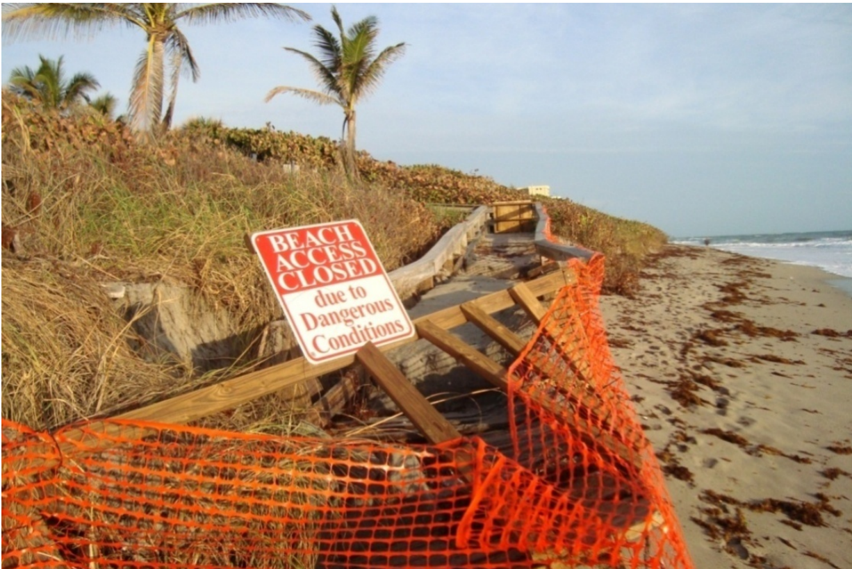
Photo (above): Jupiter beach access damaged by erosion, Nathan Schaeffer, Calvin, Giordano and Associates, Inc. ( 2011).
