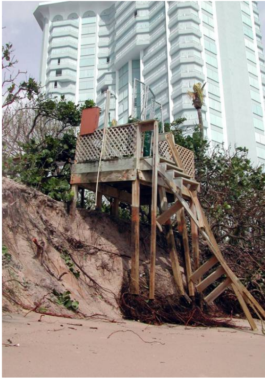
Photo (above): Damage to the Singer Island shoreline in Palm Beach County, Florida after Hurricane Frances. Courtesy of the Department of Environmental Resources Management for Palm Beach County (October 2004).
