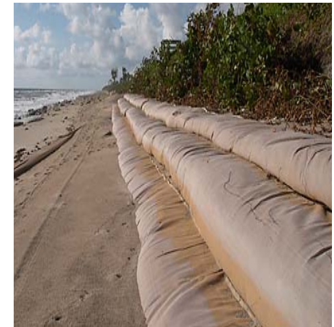
Photo (above) : Shoreline protection in Palm Beach County, Florida after Hurricane Frances. Courtesy of the Department of Environmental Resources Management for Palm Beach County, October 2004.
