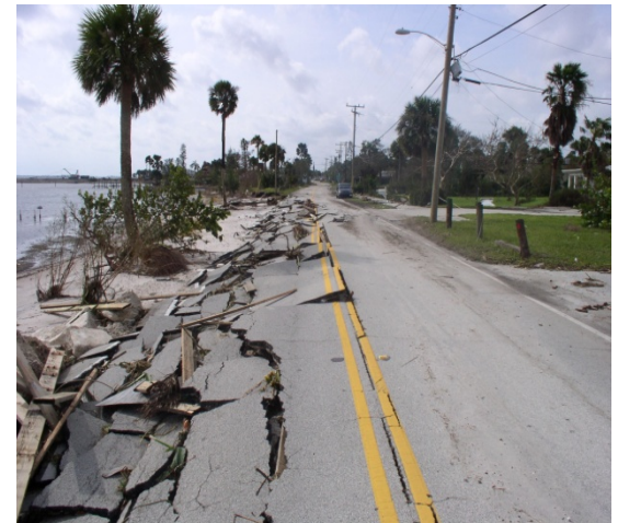
Photo (above): County Road 707 in Martin County, Florida damaged during Hurricane Frances. Photo courtesy of the Martin County Board of County Commission (October 2004).
