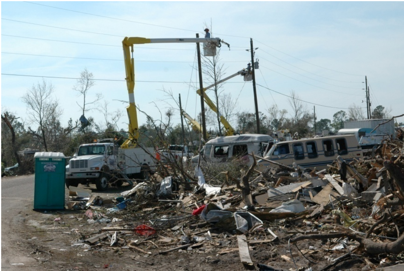
Photo (above): Lake County, FL, - Power company employees work to restore power in Lake County. The central Florida tornadoes devastated this and other areas in the county. Mark Wolfe/FEMA (February 9, 2007).
