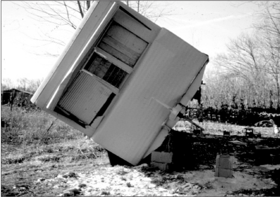
Figure 7-8. Failed foundation system that used masonry piers.
