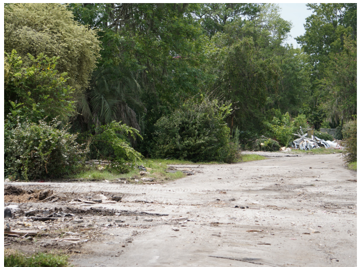
Demolition took place in July 2019, following multiple years of catastrophic flooding in the neighborhood.
