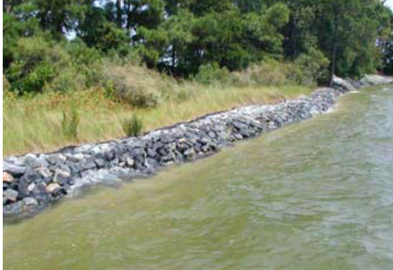
“marsh toe revetment”
