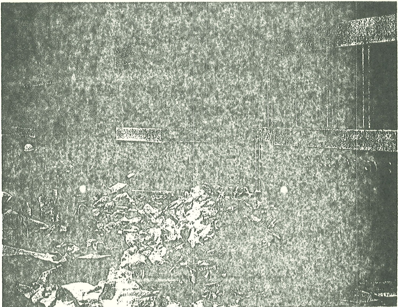
Figure 6. Key public facilities in floodplain, such as this substation and computer center of Mississippi Power and Light, required costly sandbagging. Many were disabled. (Photo by the author)
