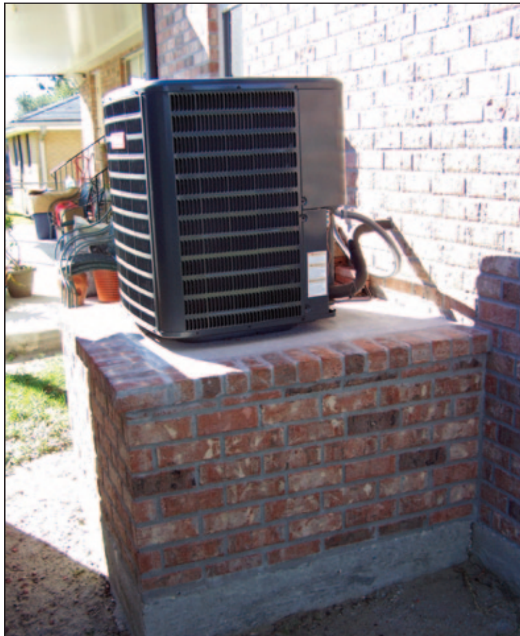
Figure 5W-1. Elevated air conditioning compressor
