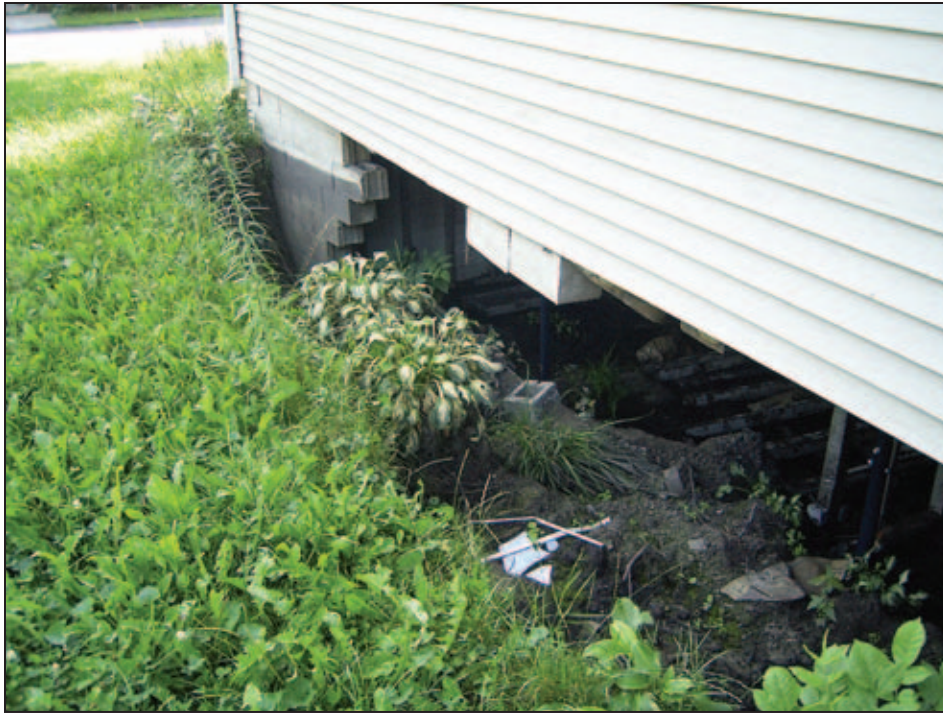
Figure 5D-29. Foundation wall failure due to pumping out basement while ground was still saturated with water
