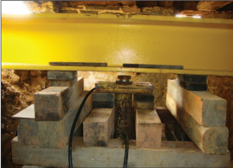
Figure 5R-7. Hydraulic jacks installed to lift structure from foundation (photo courtesy of Wolfe House Movers)
