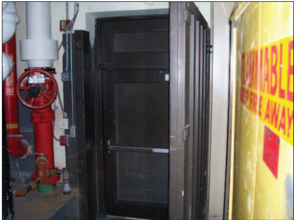
Figure 5D-38. A watertight door used to protect mechanical rooms for a hospital subject to floodwaters
