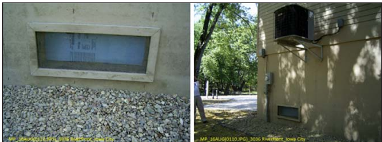
Figure 5E-14. A house where flood openings have been covered by insulation and drywall
