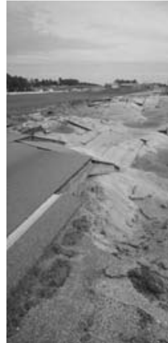
Texas road damage from flooding. Photo: FEMA
